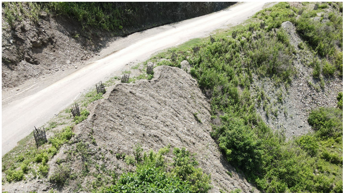
Photograph 1: Landslide and road plantation in Ramechhap. Source: tdh drone imaging (2022).
